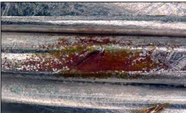
Figure 1-2 - Red Plague (Cuprous Oxide Corrosion)
